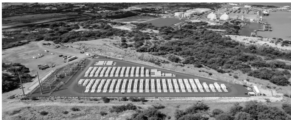
Kapolei Energy Storage
