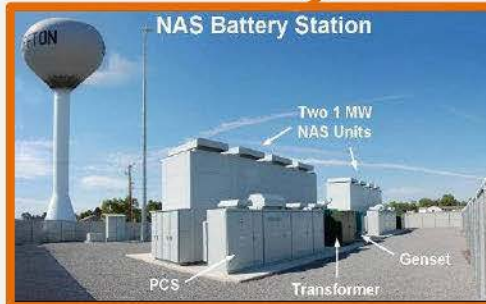
Distribution Bulk Storage 10's of MW (NaS, Li-Ion, Lead Acid)
