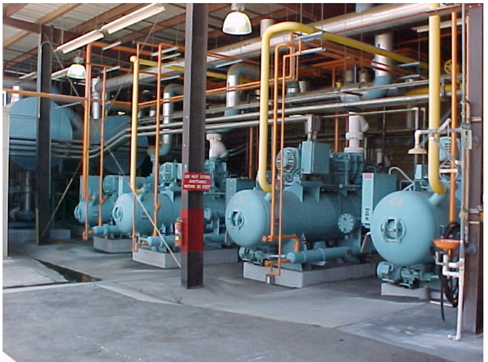
Large “built-up” industrial refrigeration plant (ASW Engineering)
